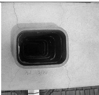
Clay Tile Liner Flue
