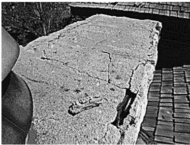
Damaged Chimney Cap
